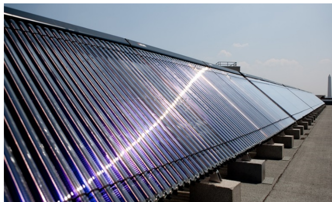
Figure 5: Solar Water Heating Panels Example
